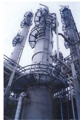
Fig. 1 – Typical industrial process columns.
