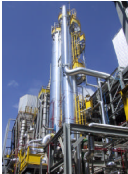
Figure 1. Distillation columns in chemical plant.
