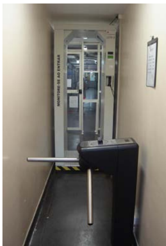
(a) Portal monitor and magnetic badge Bi-directional Barrier Arm Turnstiles for access control system - entry.
