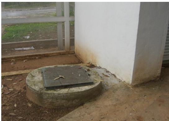
E1 point sewer pipe entrance
