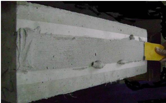
Fig. 3 The adhesive is spread over the area of bonding the reinforcement sheet.
