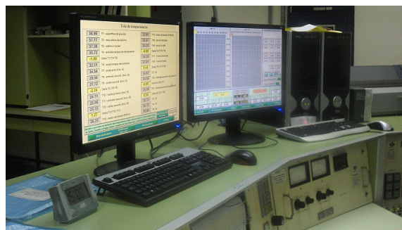
Fig. 3. Data Bank system (control room)
