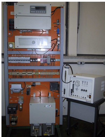
FIG. 2. Gas Analyzer equipment, model Radas 2 associated with a Gas Sampling Unit, model CFP-306 made by Hartman Braun and Shimadzu, respectively, installed in the laboratory facility for electron beam flue gas treatment at IPEN.
