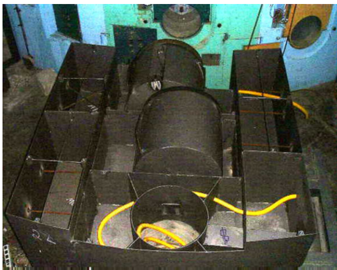
Fig. 6. Photograph of the beam shutter took during its installation in the second layer of the main neutron shield.
